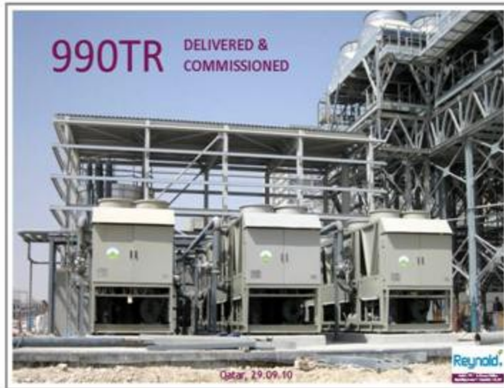
990 TR at Qatar for process cooling
